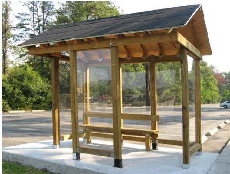
Completed bus shelter at the Metro Route 86 bus stop on Ella Blvd. A job well done. Thanks Daniel Wolf.
